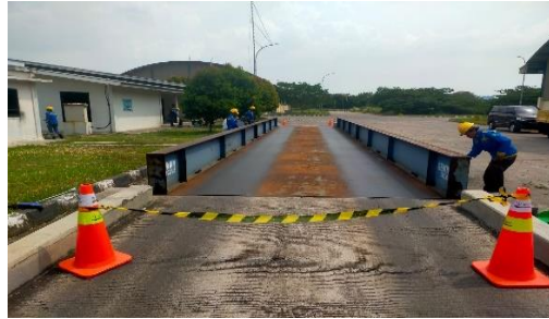
Gambar 7. Cone and Safety Lane Sumber: (PT Cahyo Permata Abadi, 2024)
